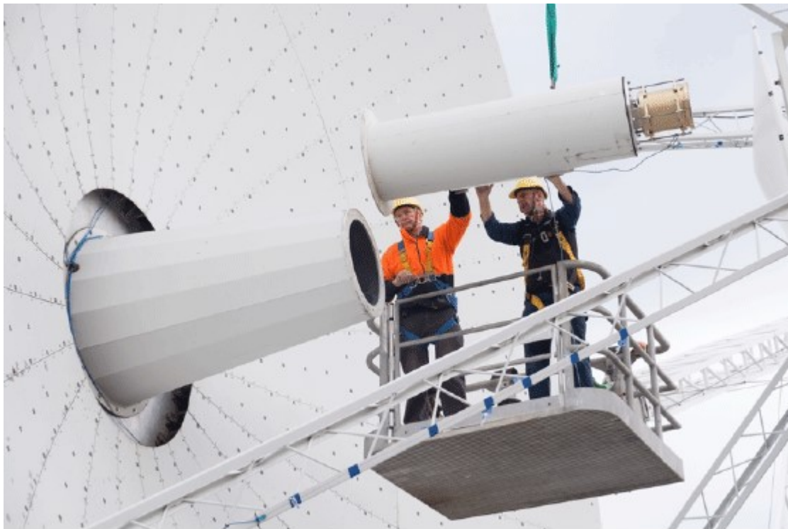
The Callisto receiver during installation at Mt Pleasant
